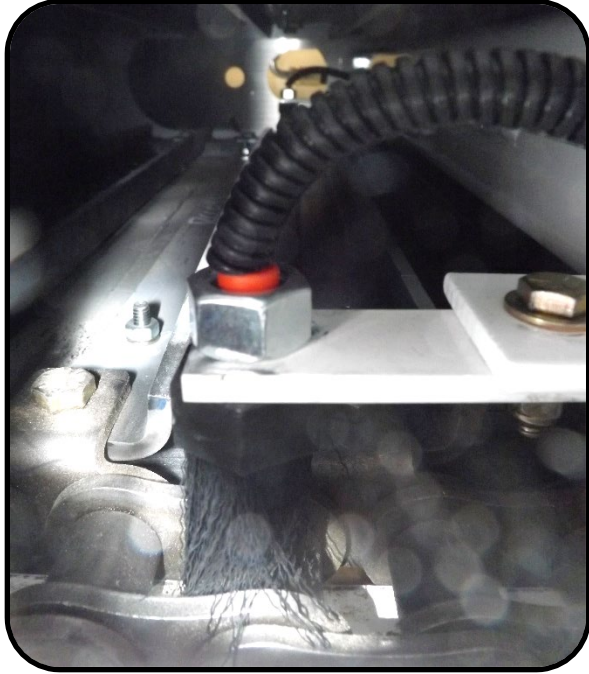
Maintenance 16. Conveyor chain brush check.
