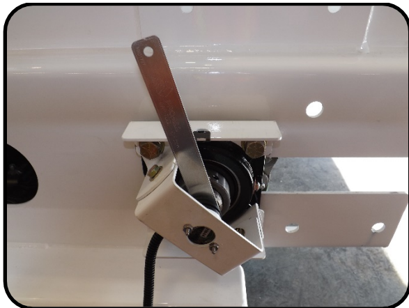
Figure 28. Speed sensor gap on conveyor drive shaft shown using a gap tool.
