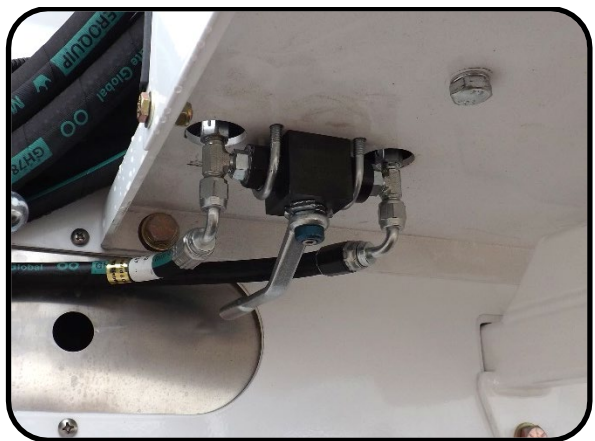
Valve Location 9. Free swing selector valve.
