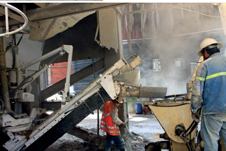
Left: The mixer uses a high-speed auger to complete the concrete mixing process. Above left: The job site featured a testing lab where samples were constantly being cured and tested.
